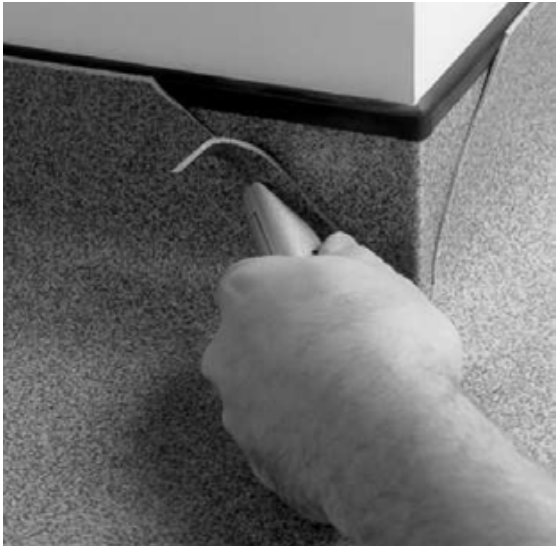
3. Using an Altro hook blade or concave blade trim the field material to fit net to the perimeter of the butterfly corner fill. Ensure the field material is held firmly down against the cove former while making the final cut.
